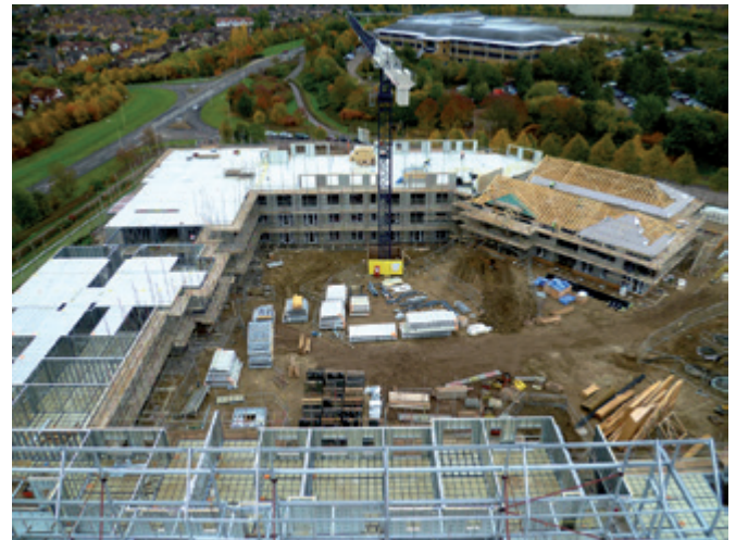
Figure 2 Construction of a light steel residential development (Image courtesy of Kingspan Profiles & Sections)
