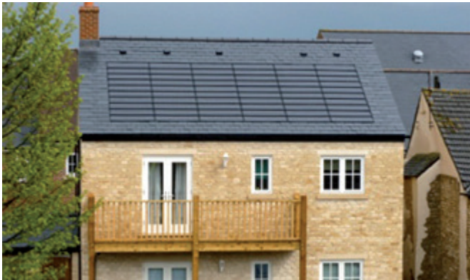
Figure 8 Photo-voltaic roof tiles on a light steel building (Image courtesy of Fusion Building Systems)
