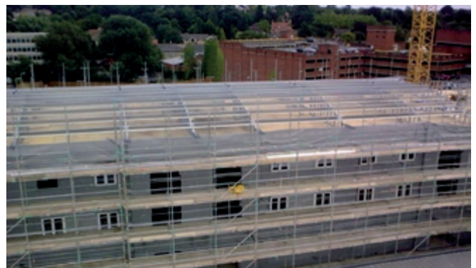
Figure 11 Light steel sections supported on cross-walls to form a curved roof (Image courtesy of Metek UK)
